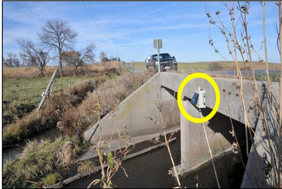
Figure 1.2: USBS installed on a Bridge crossing at Buffalo Creek, Johnson County. (Photo Courtesy of Iowa Flood Center)
